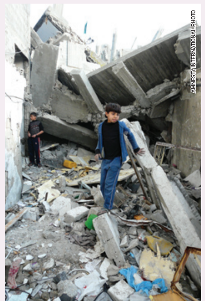
Gaza, 29 December 2008. The home of the Ba'alusha family after the next-door mosque was bombed in the middle of the night, killing five sisters Jawaher, Dina, Samar, Ikram and Tahrir Ba'alusha, aged 4 to 17, in their sleep.
